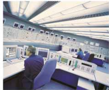
Customer switch room
